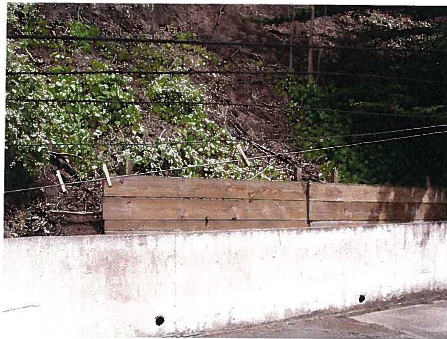
Picture #9: Retaining wall augmented to catch debris flow.
