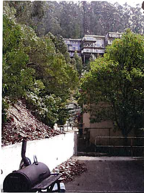
Picture #10: Debris falling over retaining wall into backyard (next to BBQ/smoker)
