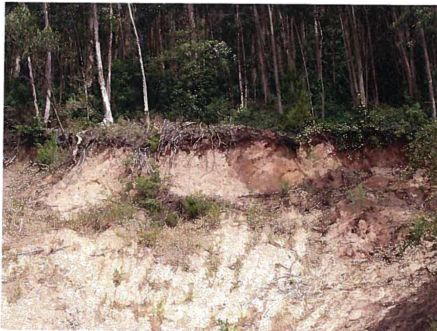
Picture #13: Existing erosion. Note exposed roots. Potential for mudslides with next heavy rain.
