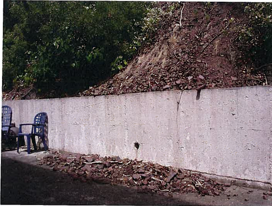
Picture #8: Debris flowing downhill behind Kirkham Heights building.
