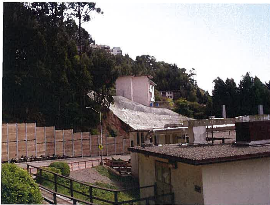
Picture #11: Retaining walls and concrete supported with rock bolts at base of Mt. Sutro
